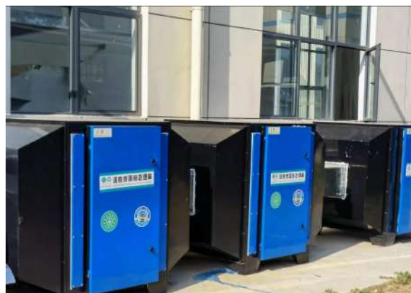
1#辅助车间废气干式过滤+二级活性炭
