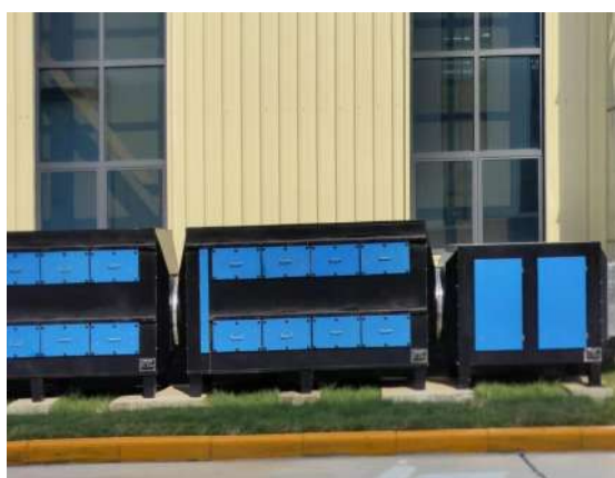
2#车间熔接和喷胶废气过滤+二级活性炭
