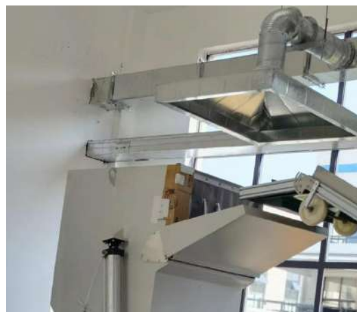
1#辅助车间破碎废气集气罩
